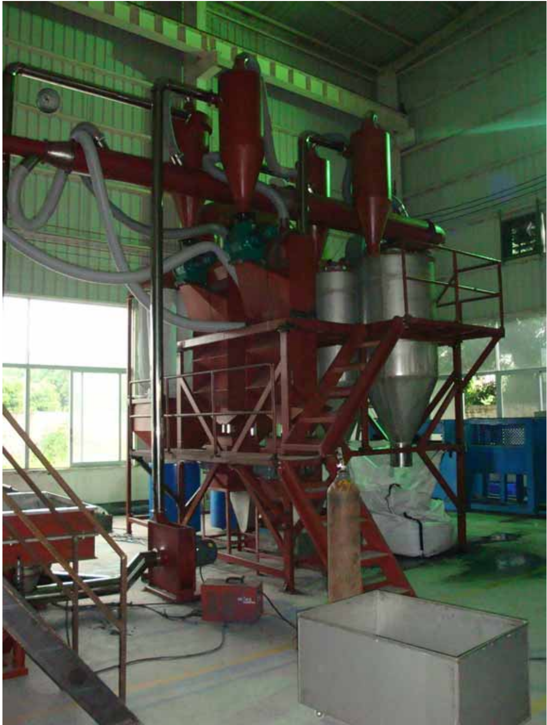
FINISHED VIEW OF THE FIBER REMOVAL SYSTEM AND FINE MAGNETIC REMOVAL SYSTEM AND CYCLONE SYSTEM AND GRAVITY SEPARATION
